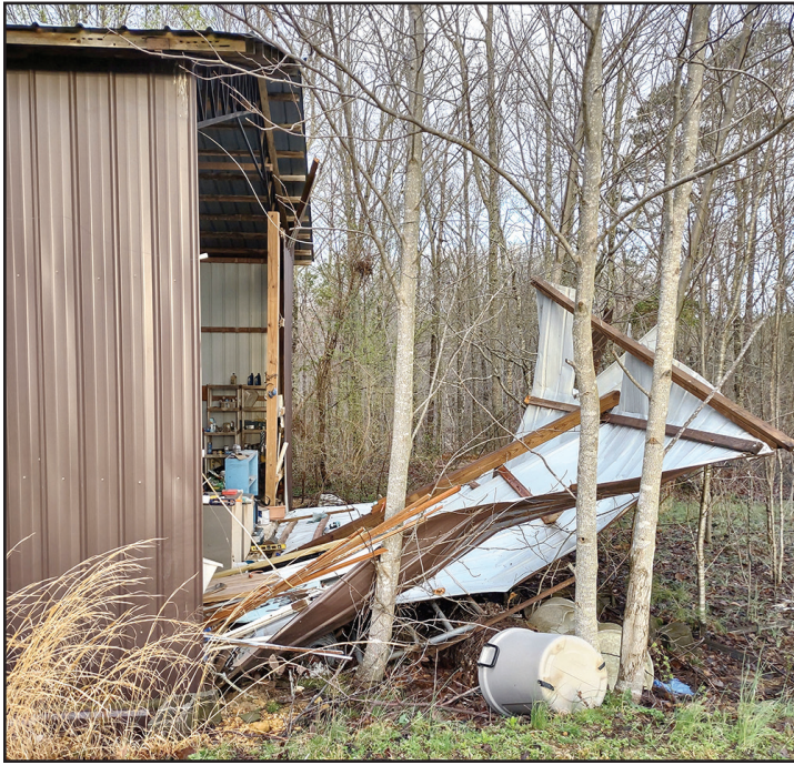
This outbuilding on Kilburn Hollow Road had a back wall that was completely blown out by the wind last Tuesday.
