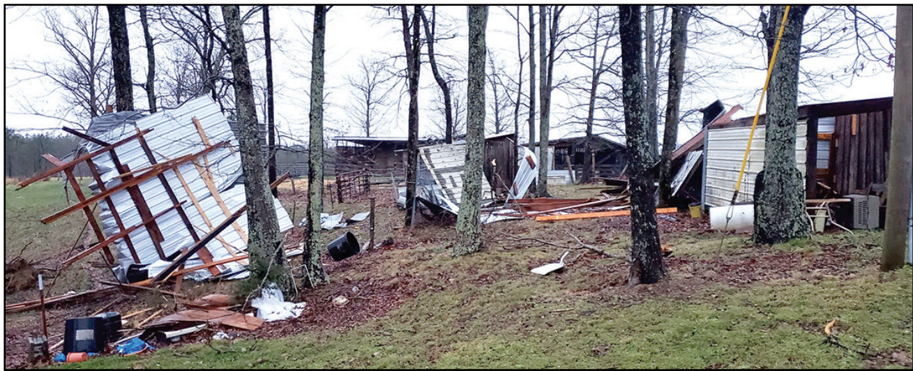
Some sheds and outbuildings sustained heavy damage at a residence on Sherrill Drive in Waynesboro during the winds last Tuesday.
