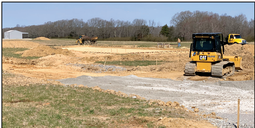
Progress is being made at the new Ag Center facility at the Wayne County Industrial Park on Highway 13 South. It was reported at the commission meeting that crews are working on the concrete and plumbing for the facility at this time.
